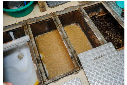
Commercial Kitchen Grease Interceptor
