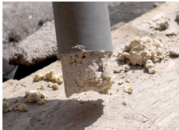
Pipe clogged with fats, oil and grease
